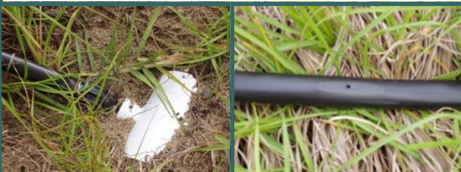
The Newly Installed Netafim USA Irrigation System
