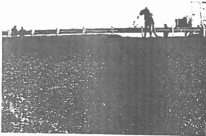
Band-Aid for construction scar
