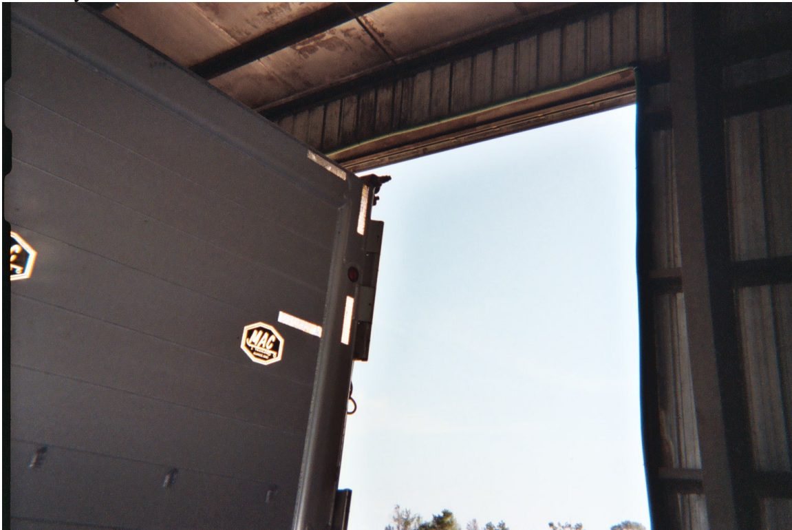
Figure 2 – MSW Tipping Building Distribution Hose Attached to Sides & Top of Doorway
